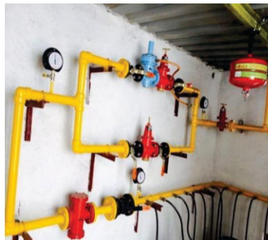
LPG Manifold System KEPL-100
